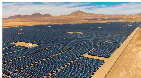
CFV Puerto Peñasco, the largest solar power plant in LATAM | CFE.
