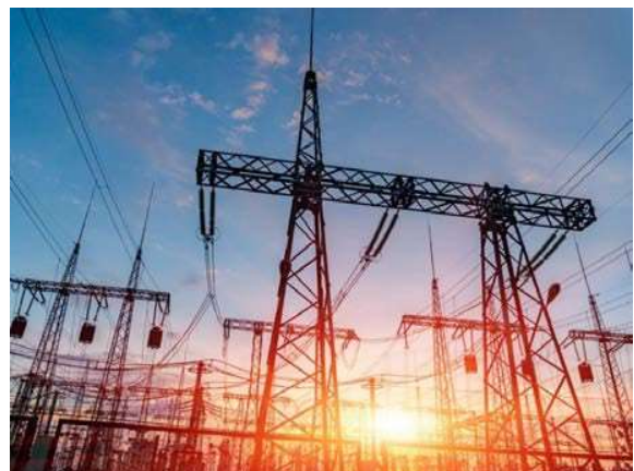
Transmission Substation | CFE.
